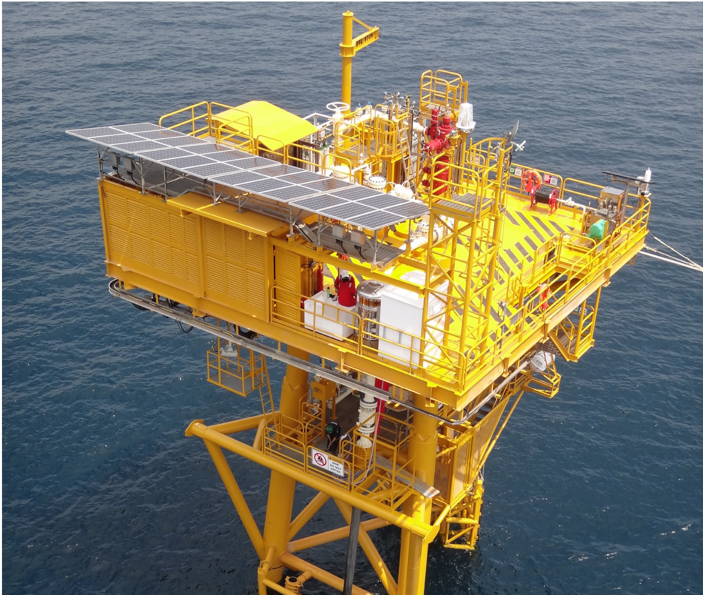
Panel surya di Platform Wellhead Peluang, Madura Offshore, Jawa Timur, Indonesia
